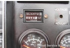
© Diesel Service & Supply
